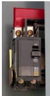
QO2100 Tenant Circuit Breaker Installed
