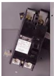
Q2M2200VH Tenant Circuit Breaker Installed
