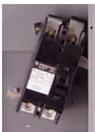
Q2M2200VH Tenant Circuit Breaker Installed
