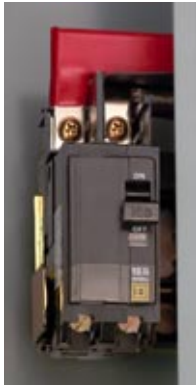
QO2100 Plug-On Circuit Breaker Installed
