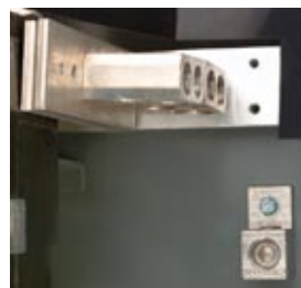
Ground Lug and Isolated Main Neutral Bus as Installed at Factory on Main Devices
