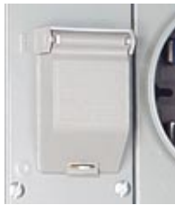
Circuit Breaker Cover, Closed
