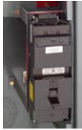
QE3200VH Tenant Circuit Breaker Installed
