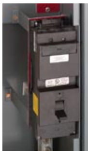
QE2200VH Tenant Circuit Breaker Installed
