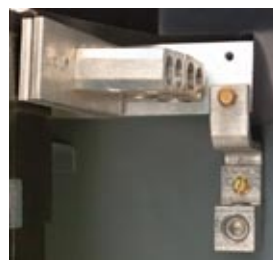
Service Ground Lug, Bonding Strap and Bonded Main Neutral Bus as Installed on Main Devices at Job Site as Required for Use as Service Equipment
