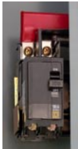
QO2100 Tenant Circuit Breaker Installed
