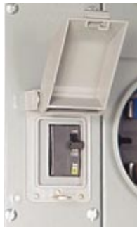
Circuit Breaker Cover, Open
